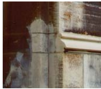
Black crust that was 1/4" thick removed from the Cathedral of Learning at the University of Pittsburgh with one application of Stripper Cream in one hour.
