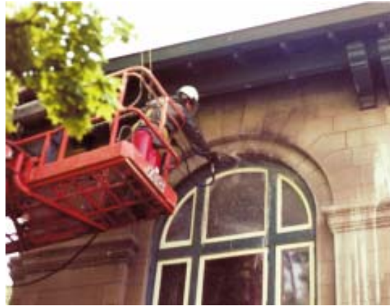
Limestone restoration at the Monroe County Historical Society's building in the heart of Indiana's limestone country. The area of black in the arch is not yet rinsed, but has been treated with SafeRestore.
