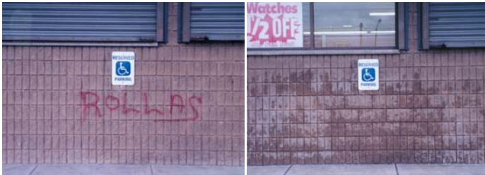
Before and after of graffiti removed from porous concrete block wall leaving no shadow.
