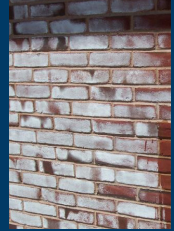
Efflorescence (calcium chloride)
